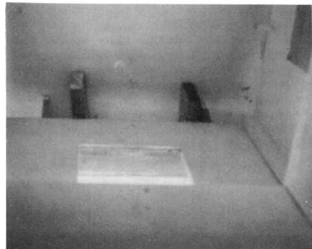
Fig. F.4. View from Below the Exit, Looking Up the Multi-Purpose Emergency Exit Housing. The top is shown supported in a tilted position by two 6-inch-wide boards placed between a wall and the top.
