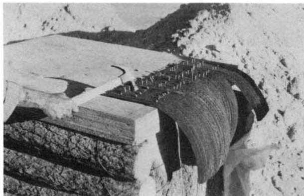
Fig. D.15. Tire-strip hinges nailed to an expedient, 4-inch-thick blast door made of plywood, designed to withstand 50-psi blast effects of very large weapons and undamaged by blast at the 53-psi range.
